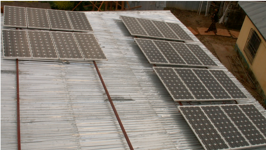
Figure 11.1: 24 solar panels with a nominal power of 80 W have been mounted to the roof of the NOC to provide power to the system 24/7.
