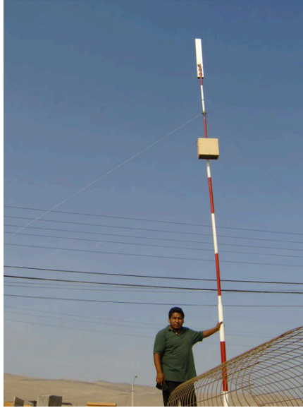
Figure 11.20: Quiani node. This is one of the world's highest nodes. Its located at an elevation of 4000 m, about 2000 km north of the country's capital.
