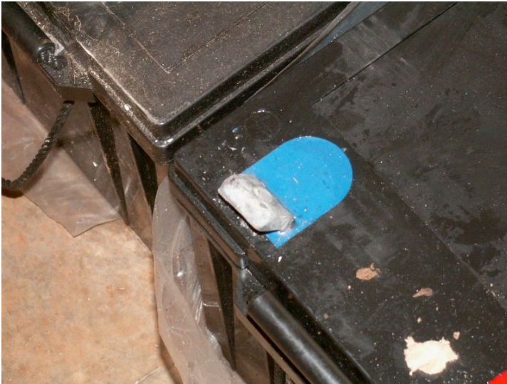
Figure 7.2: A 200 Ah lead-acid battery. The negative terminal was broken due to weight on the terminals during transportation.
