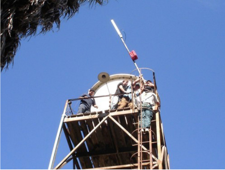
Figure 11.24: Implementation of node over a water tower in Batuco, Metropolitan Region, providing backhaul to Cabrati telecenter.
